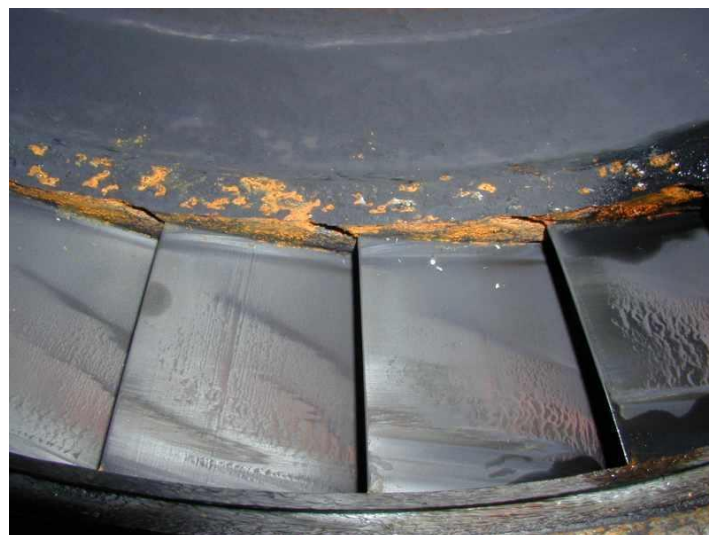
Figure 42 Turbine Blade Erosion and Corrosion
